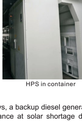
HPS in container
